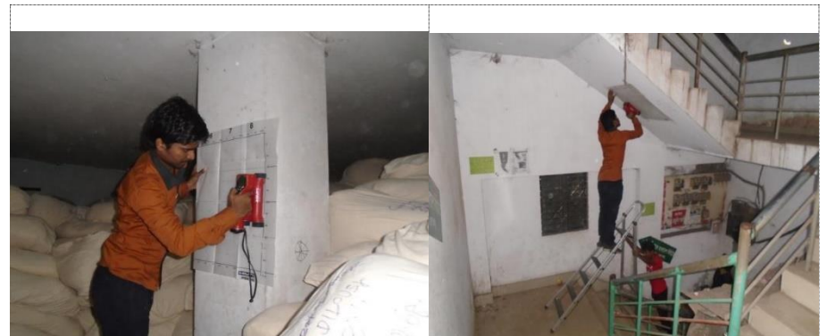
FIGURE: - RE-BAR SCAN FOR DIFFERENT ELEMENT OF STRUCTURE (BAY CREATION LIMITED, NARAYANGANJ)
